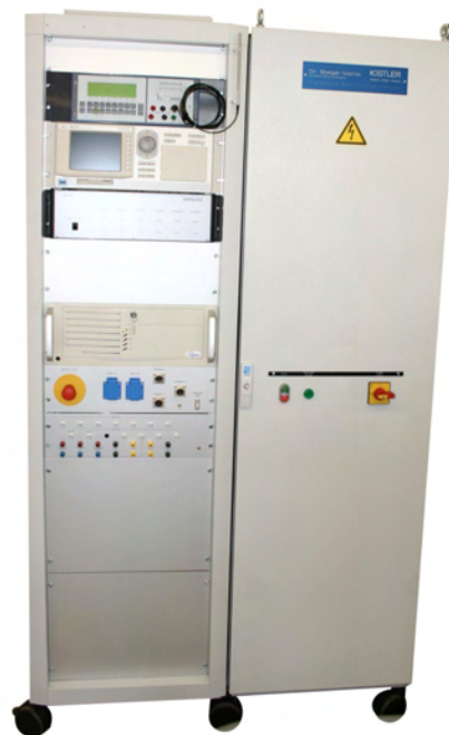
Fig. 3: Measuring equipment control cabinet
